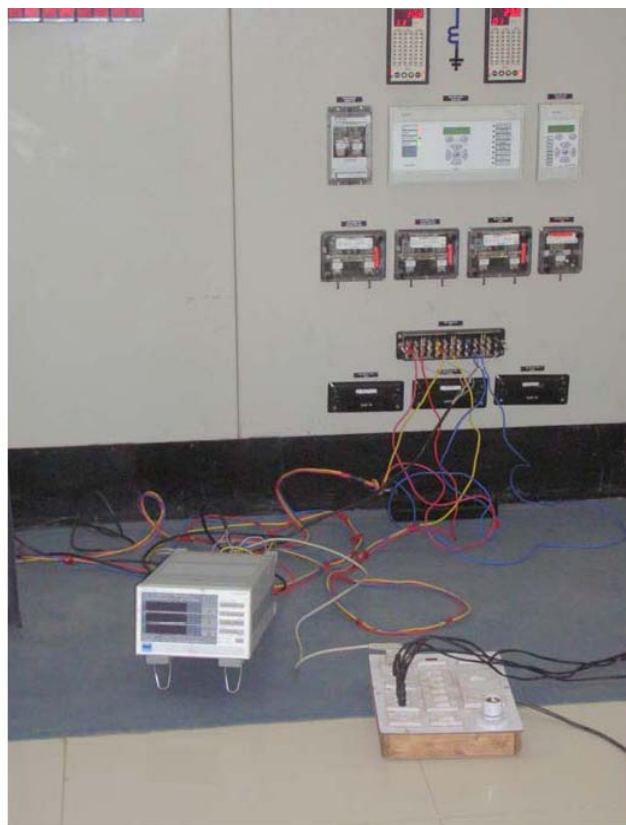
Fig. 36 : Reference meter connected at TTB without opening the control panel
