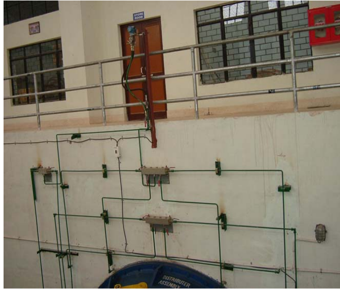
Fig 30 : Upward sloping pipes and valves for purging
